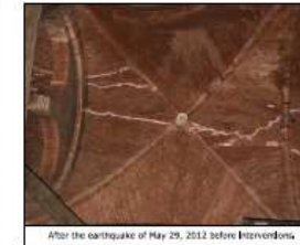
After the earthquake of May 29, 2012 before Interventions
