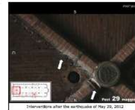
Interventions after the earthquake of May 29, 2012
