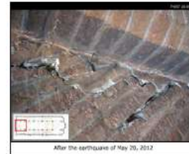
After the earthquake of May 20, 2012
